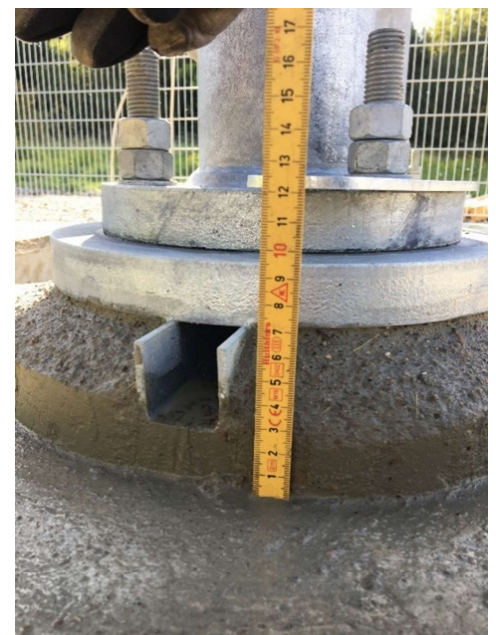
Example of under casting
