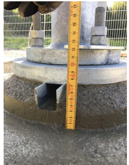
Example of under casting
