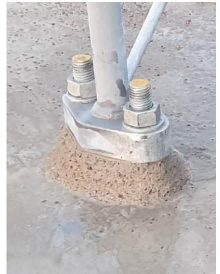
Example of under casting
